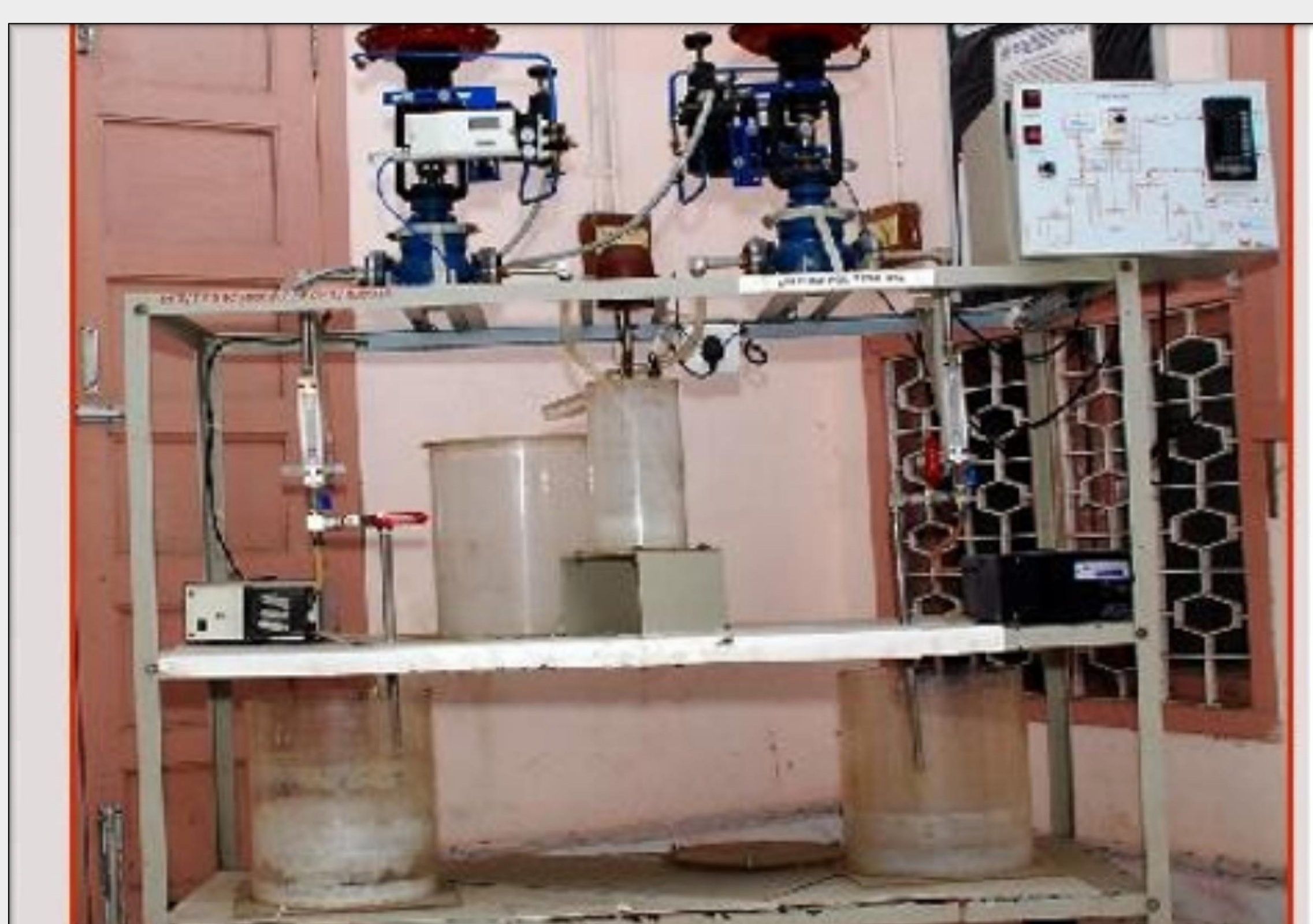
pH Control Test Rig
