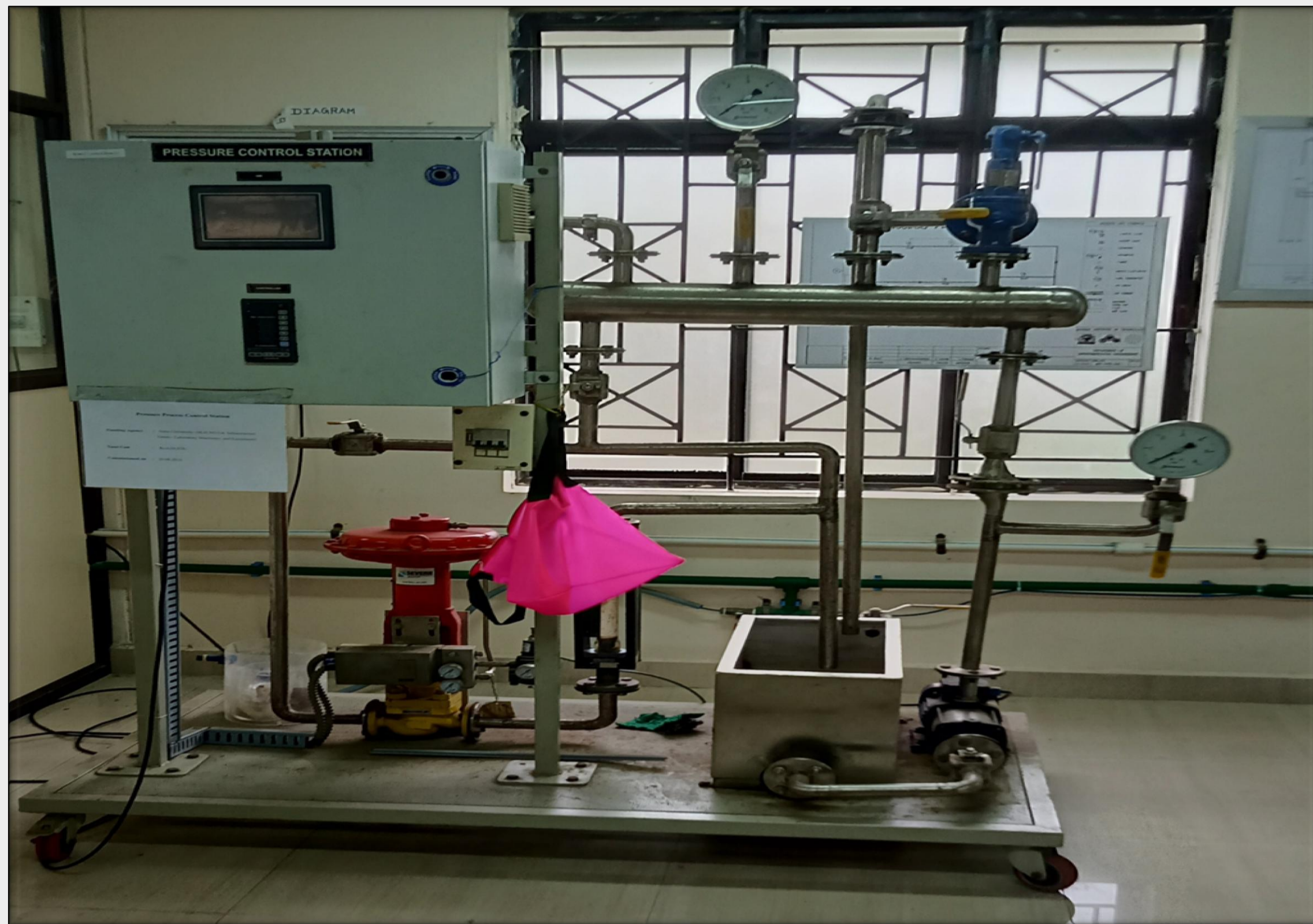
Pressure Control Station
